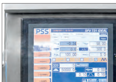
Central control panel
